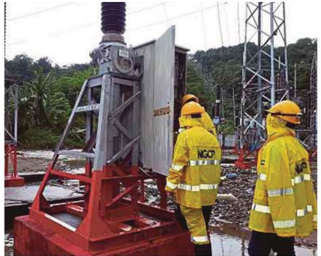
Pestech International Bhd says the Cebu-Bohol 230kV Interconnection project is its third power infrastructure deal awarded by National Grid Corp of the Philippines. WEBSITE PIC
